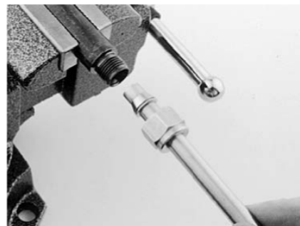
Back nut off of Pre-Setting Tool. Notice the collets have swaged into the tubing. Now take tubing to installation area.
